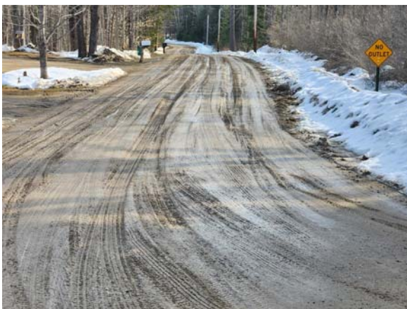
Figure 1 – Sta. 0+00 gravel roadway surface condition.
