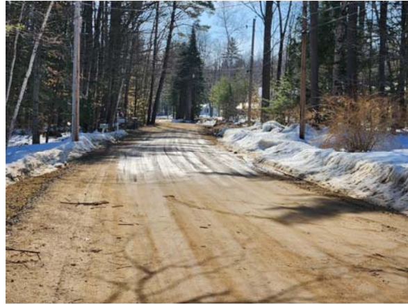
Figure 4 – Sta. 30+60 gravel roadway surface condition.
