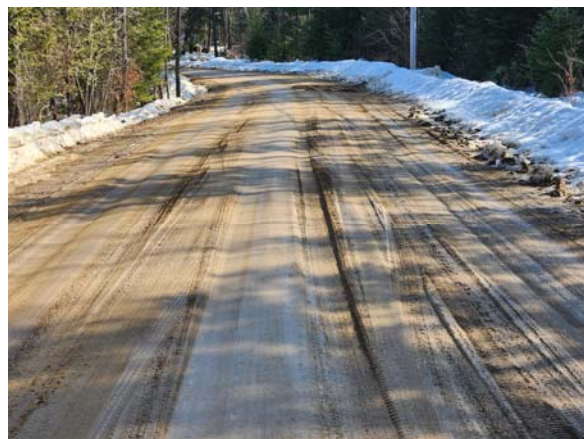
Figure 2 – Sta. 5+40 gravel roadway surface condition.
