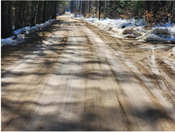
Figure 3 – Sta. 21+05 gravel roadway surface condition.
