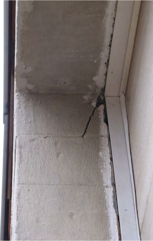
Photo 029: Crack in top of center pier between overhead doors, showing translation of block below top course.
