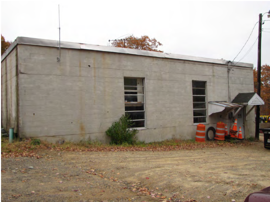
Photo 001: West wall of building. Note crack at bottom of top course of block, just below metal fascia, at southern half of wall. See detail photos 003 and 006.
