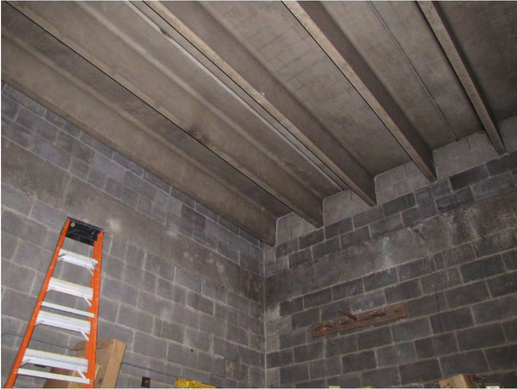
Photo 040: Typical precast concrete double tee roof framing bearing on masonry block wall at eastern 3/4 of building. Note concrete band beam two courses below bottom of tees.
