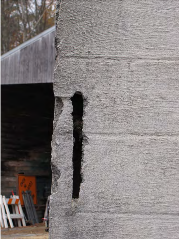
Photo 021: Deteriorated masonry with hole in face shell of south end of east wall.
