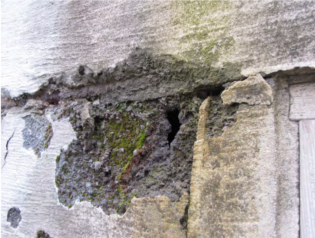
Photo 015: View of Photo 012 with knife removed. The masonry around the hole in the face shell crumbles in your hands.
