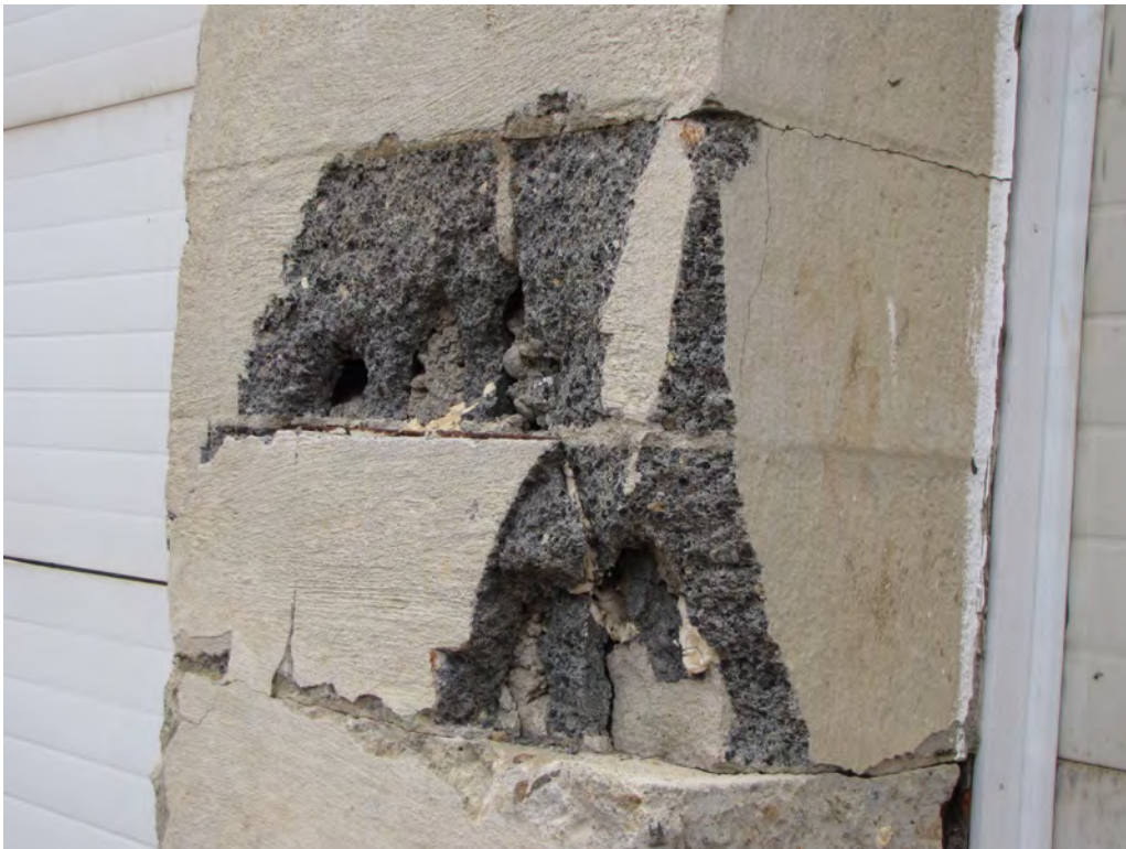
Photo 028: View of pier between two center overhead doors at top of concrete. Damage to masonry is likely due to impact by vehicles or equipment. Masonry has translated towards the inside of the building.
