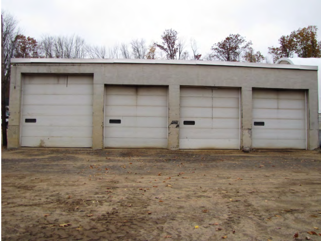
Photo 036: South face of garage building with 4 overhead doors. There is extensive structural damage to the concrete and masonry block pier between the two center doors and between the two right, or easterly, doors.
