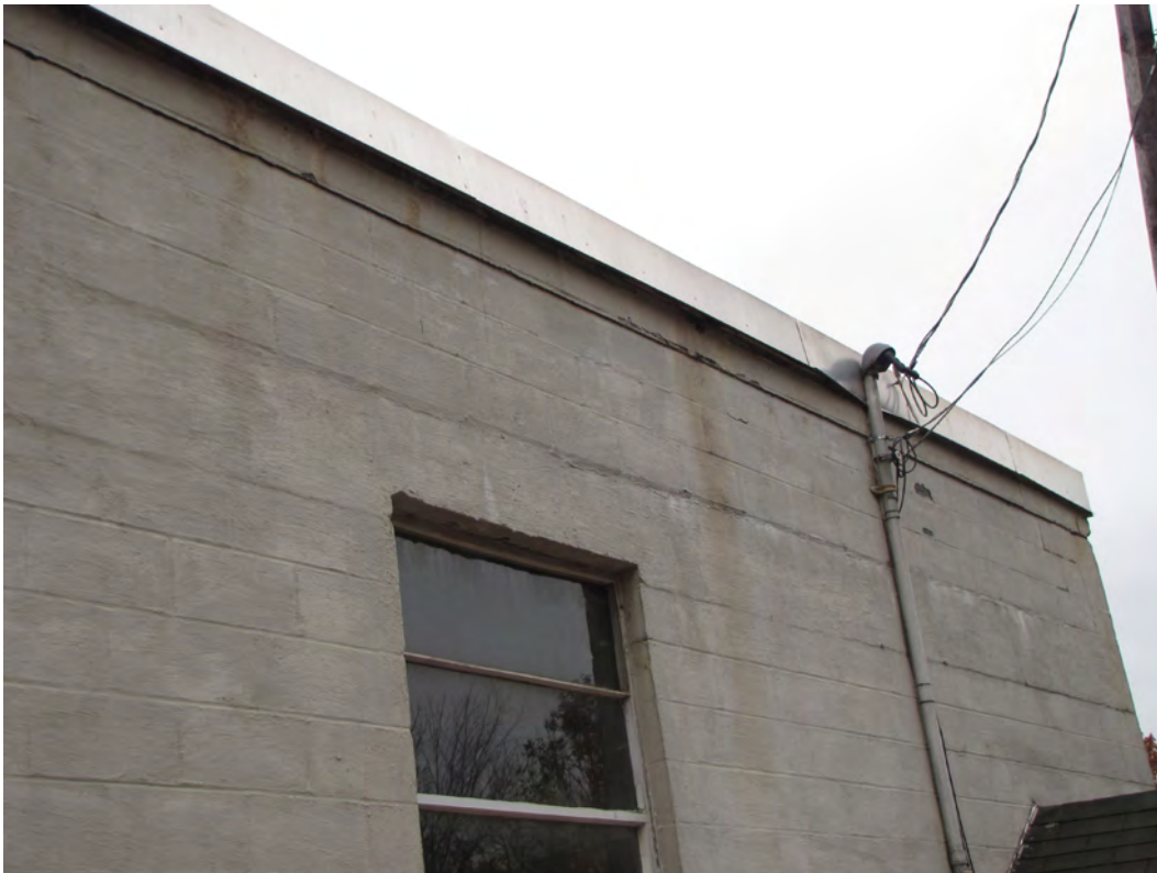
Photo 003: Closer view of south half of west wall showing top, 4 th course of masonry above concrete band beam, cracked and laterally displaced to the outside from the wall below.
