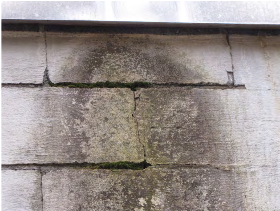
Photo 009: Water damage to north wall of building where water is overflowing roof through "scupper" created through the metal fascia. Moss is growing in mortar joints which are cracked and permit water infiltration.
