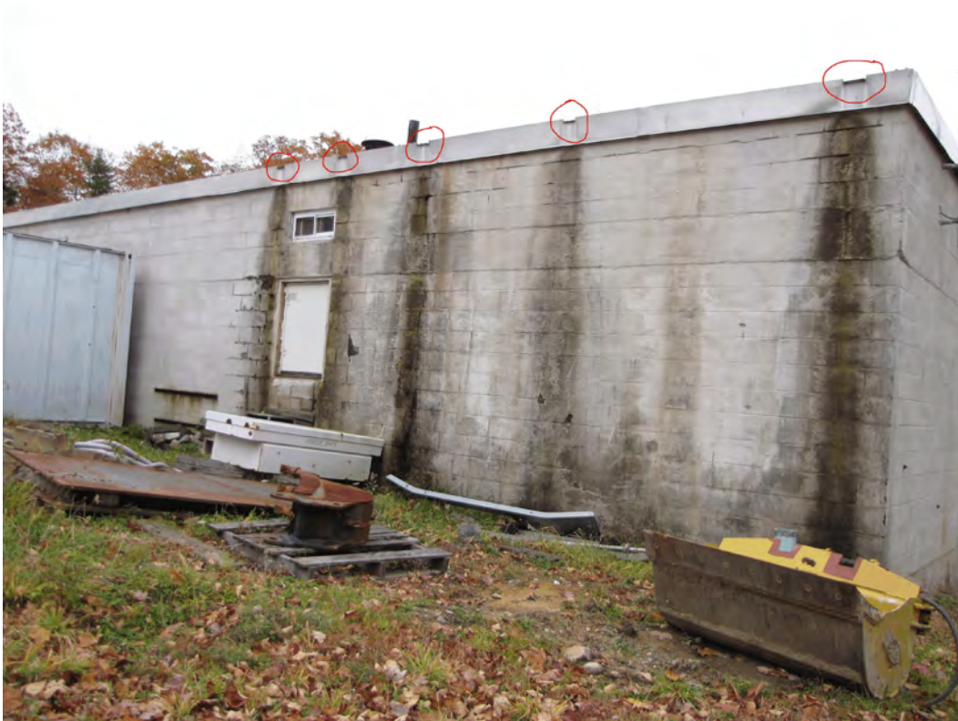
Photo 007A: North wall of building, showing effects of water runoff from roof. See detail Photos 009, 010, 011, 012, 013 and 015. Note that the metal fascia has been cut and folded down at 5 locations (in red circles) to form scuppers for roof drainage.
