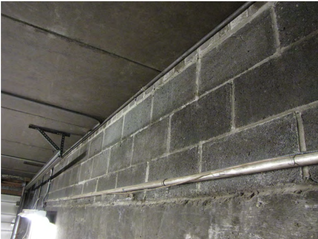
Photo 047: Typical precast concrete plank shown at west exterior bearing wall. Note there are 3 full courses of masonry blocks above the concrete band beam plus a course of concrete masonry brick.
