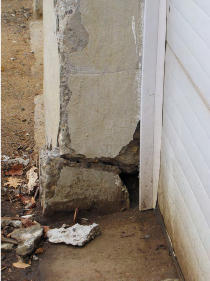
Photo 023: Close up of Photo 022A showing extreme movement of concrete pier. This structure is unreinforced concrete. The pier is unstable and not safe.
