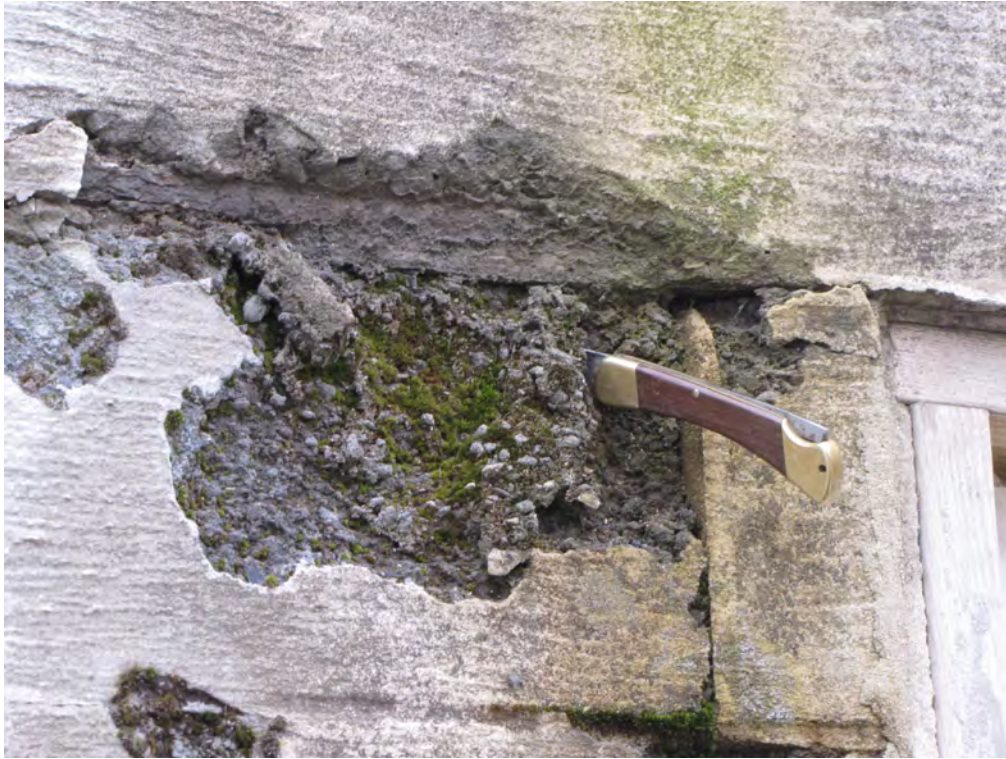
Photo 012: Close up of Photo 011 at upper corner of hatch door. Masonry is so deteriorated a dull knife blade can push right through face shell. Note the bottom outside corner of the concrete band beam is spalled off (cracked and fallen off).
