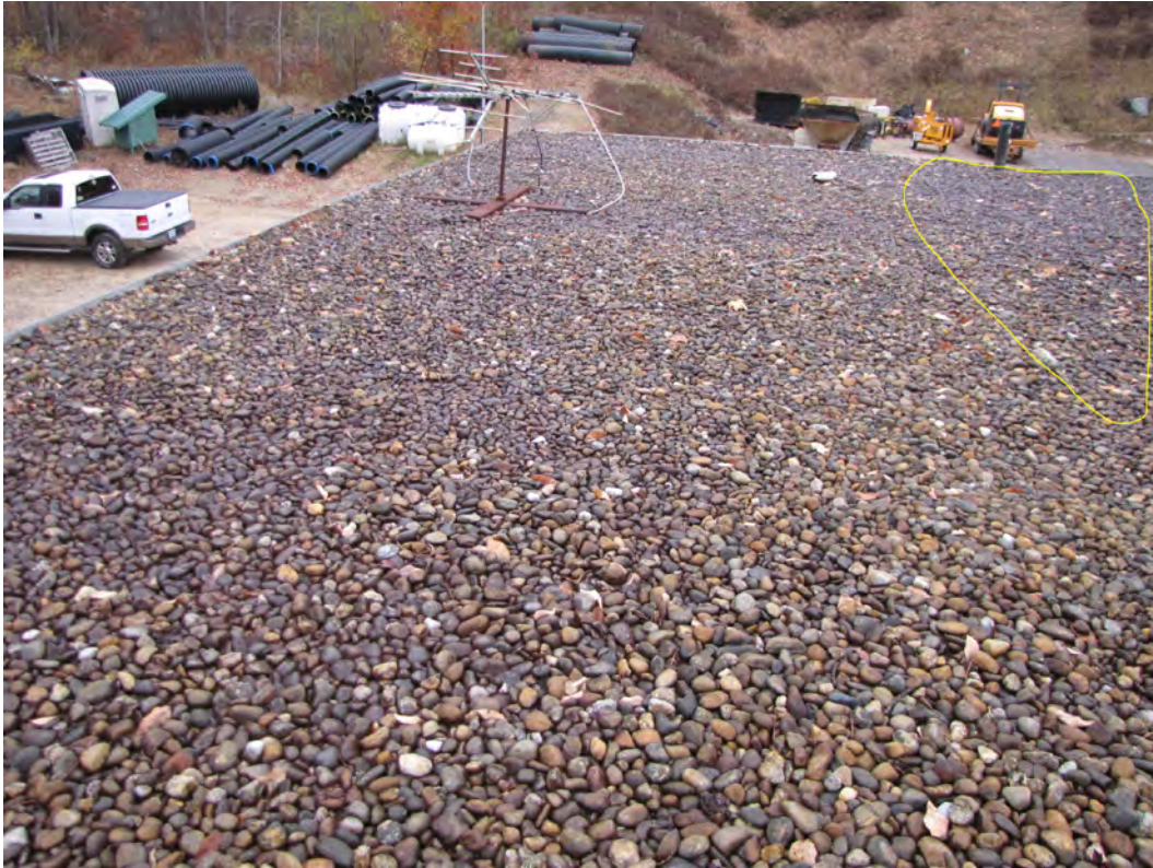
Photo 044A: General view of roof looking NW. Area of dark stone within yellow boundary has standing water on the roof.
