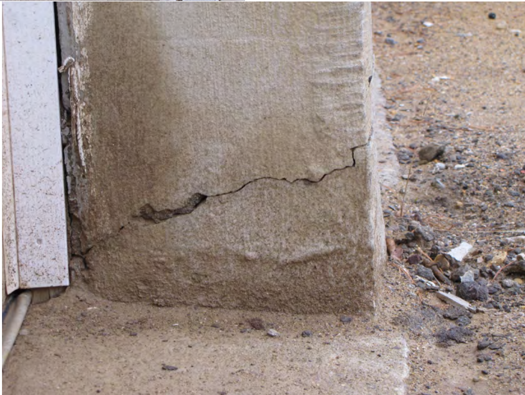
Photo 033: Crack at bottom of concrete center pier at overhead doors. Shear crack results from lateral impact force on exterior face of pier.
