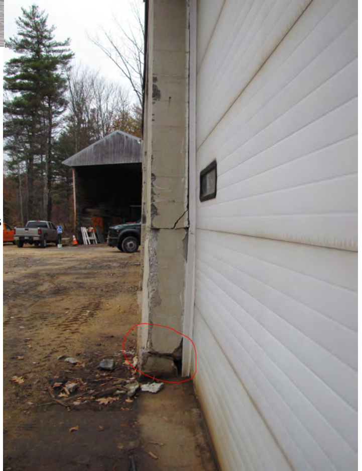
Photo 022A: South wall of building, looking west at pier between first two overhead doors. This pier was hit by a vehicle, cracking and dislodging the pier towards the inside of the building. Area in red circle has about 2" of movement.
