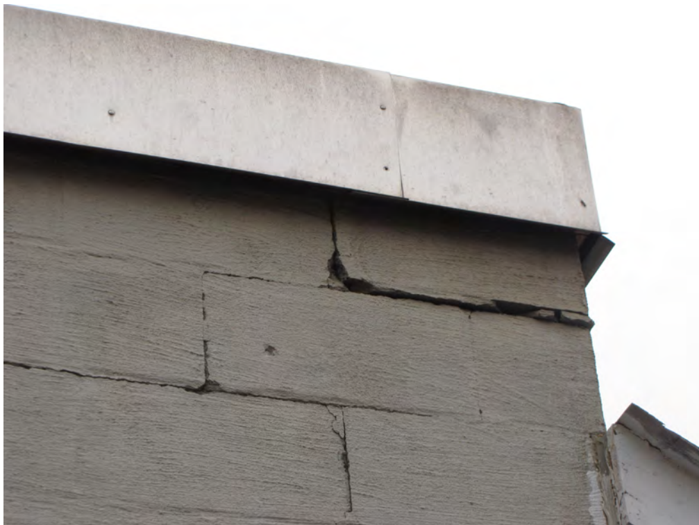
Photo 018: North end of east wall showing cracked and loose block at corner.
