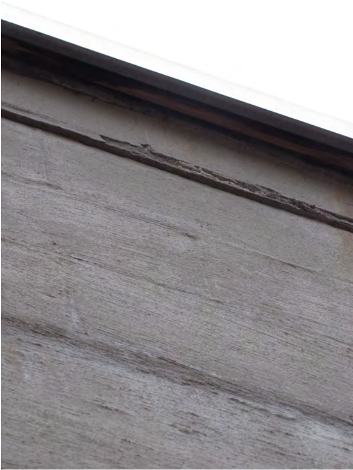
Photo 006: Close up of the west wall in Photo 003 showing about ½" of lateral displacement of the top course of masonry block. This course is located mostly at the thickness of the precast concrete plank roof inside.
