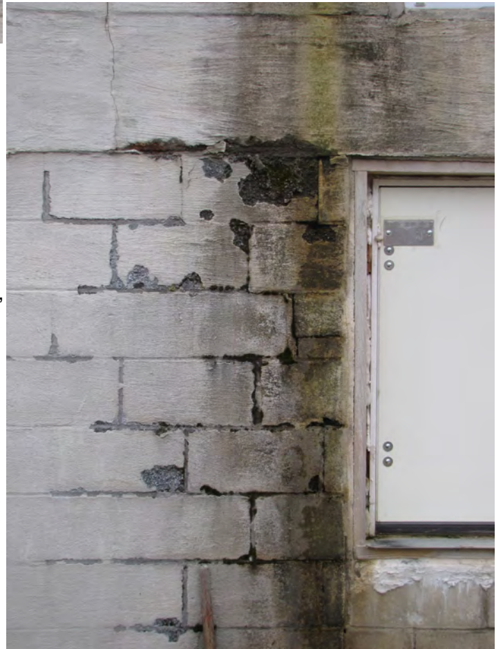
Photo 011: Significant water damage of north wall, on east side of emergency egress hatch door. Masonry is spalled and joints cracked. Note crack through concrete band beam.
