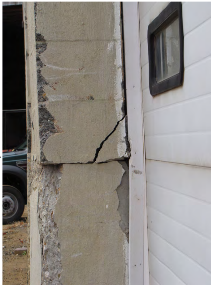
Photo 024: Joint interface closeup of concrete to block, from Photo 022A. Note position of outside face of block of this pier relative to the pier beyond.
