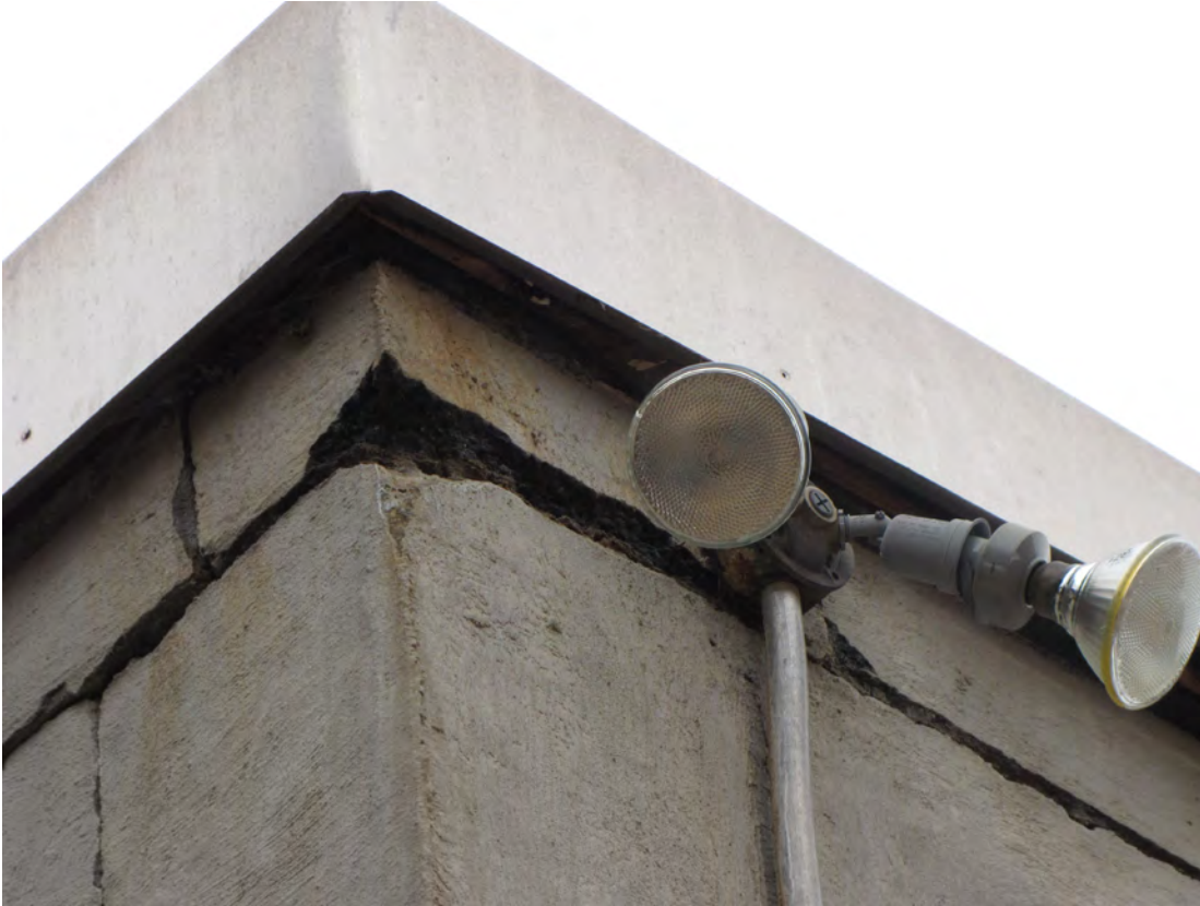
Photo 038: SW corner of building showing deterioration of block and mortar joint at top course of block.
