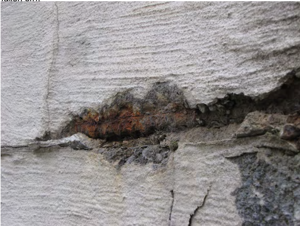
Photo 013: Close up of Photo 011 at the bottom of the crack in the concrete band beam. Reinforcing bar is visible where concrete has spalled off. There is insufficient concrete cover around the bar. Corrosion will cause continued cracking and concrete deterioration.
